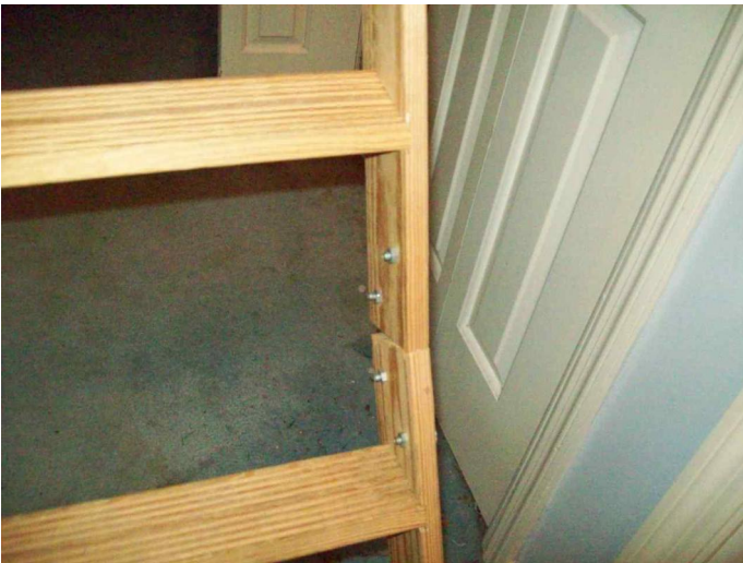
Attic pull down stairs the legs need to be cut to proper length
