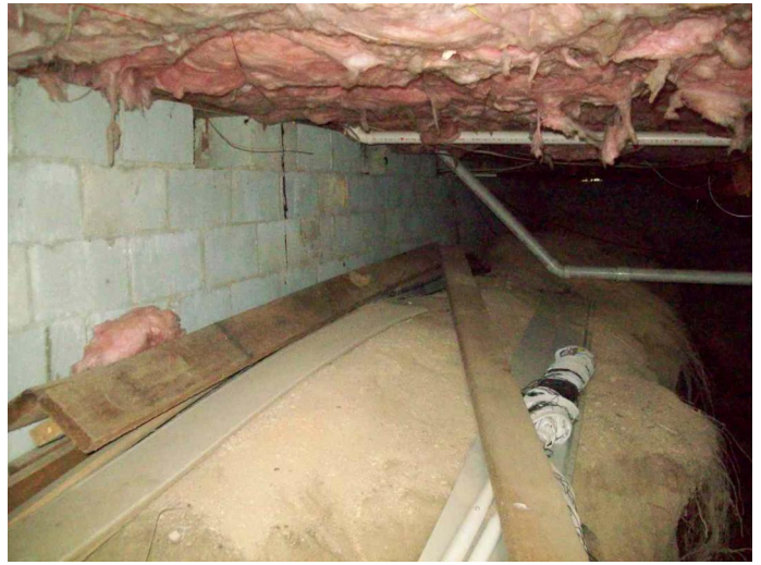
Wood to earth contact in crawl space.
