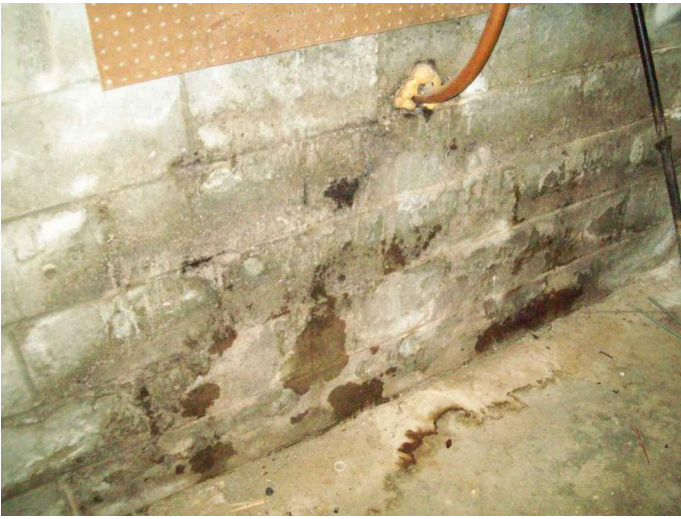
Signs of water intrusion at front foundation wall
